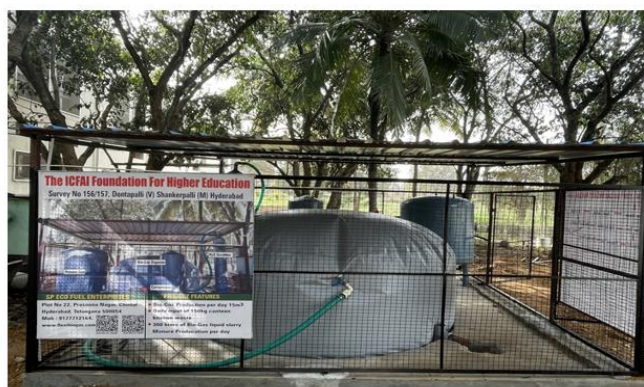
Biogas Plant on the Campus
