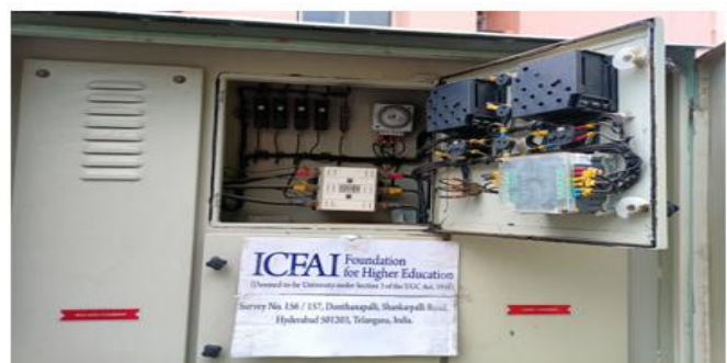
Sensor-based Feeder for Time Control for Lights
